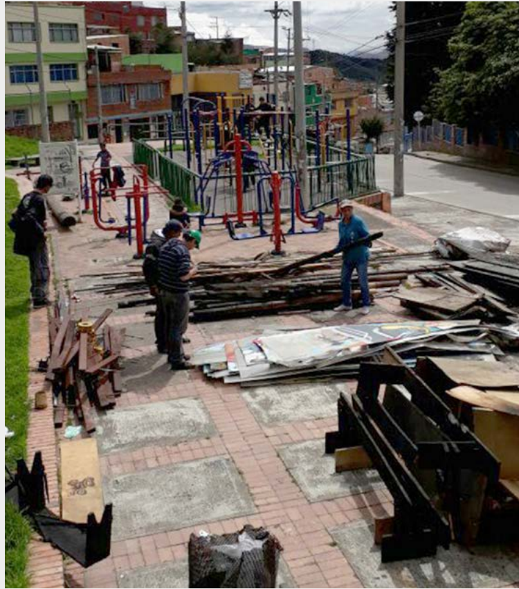
Figure 2: Sorting of materials during the disassembling of Casa del Viento. Source: Own elaboration, 2017.
